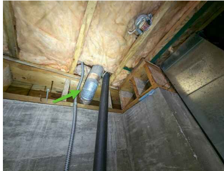
Dryer Exhaust Ducting
