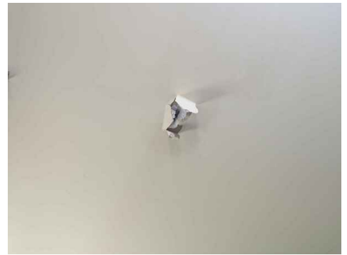
Hole in ceiling
