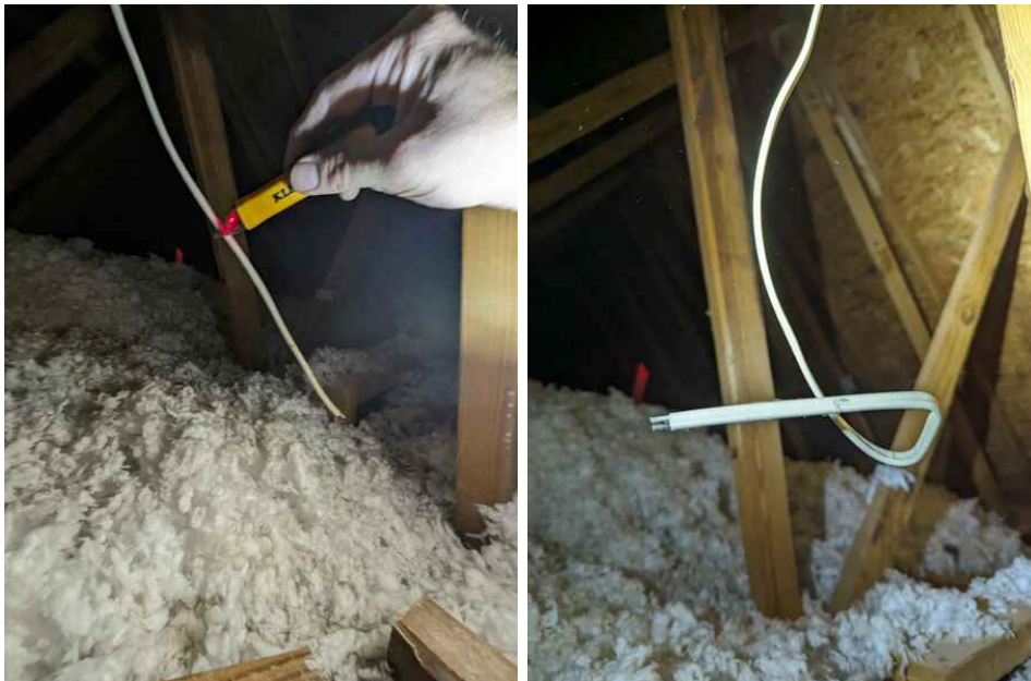
Live Electrical just inside the attic access hatch
