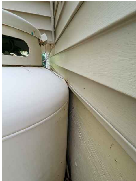
Propane Tank is touching the house.
