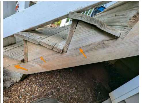
Continuous Crack running full length of right side stringer
