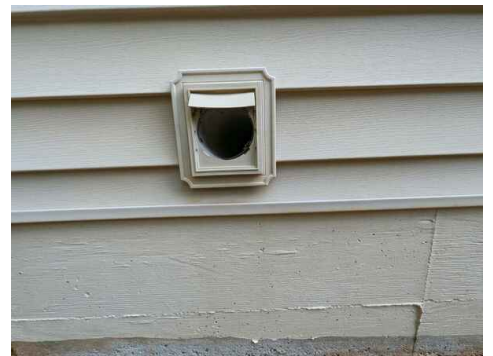
Missing or Broken Louvers on dryer exhaust vent in front of house
