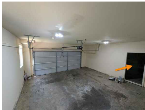
Door into Utility Room does not have a self closing hinge.
