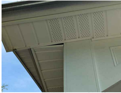
Front corner above the porch soffit is falling down.
