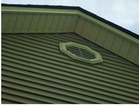
Gable End Vent
