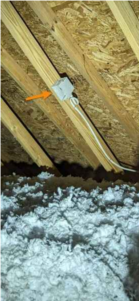
Open Junction Box
