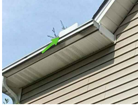
Kick out flashing garage side of front gable roof blocked by tree limb
