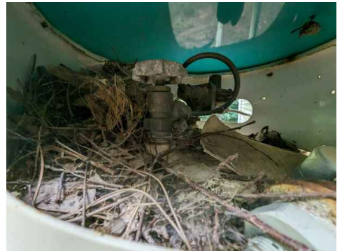
There appears to be a bird nest located inside the lid of the propane tank
