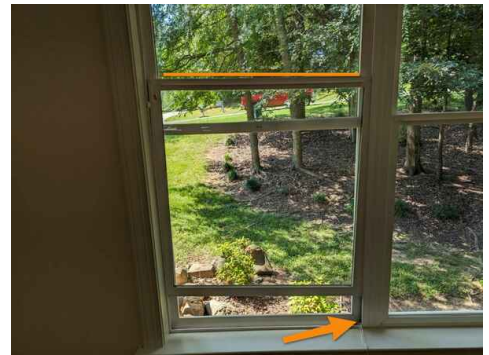
Window sash sits crooked in the frame due to broken weight.
