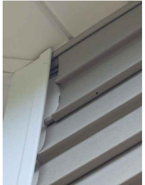
Siding does not extend all the way to the corner.
