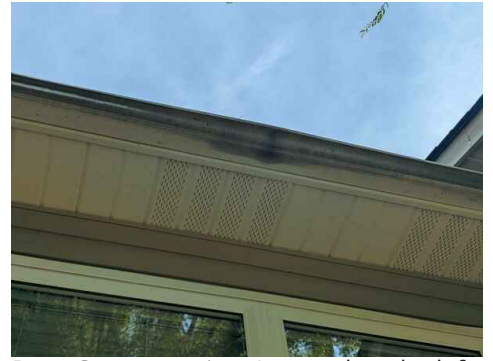
Bent Gutter section. Located to the left of the front porch.
