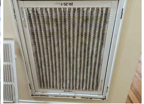
Main Stack Filter at top of stairway
