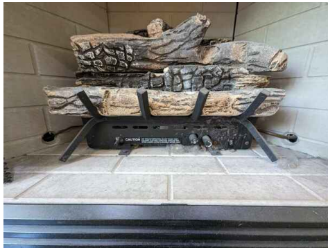
Flammable debris inside firebox
