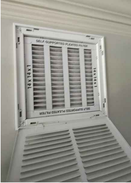
Filter in basement
