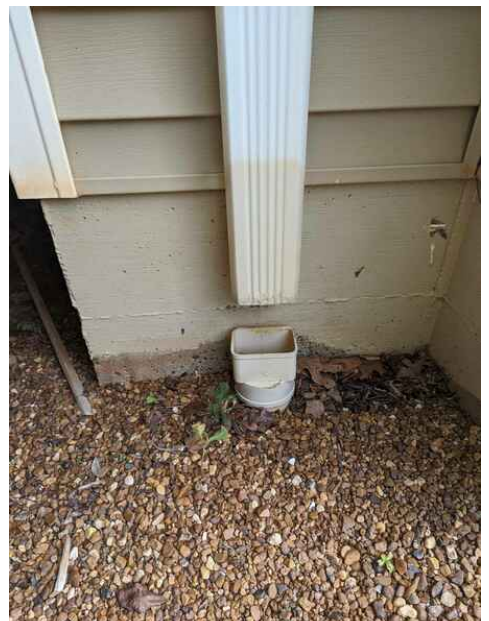
Missing Boot connecting downspout to drainage system. Located beside front porch.
