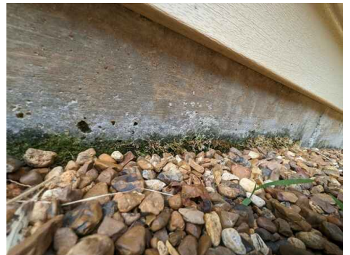
Moss growing on side of slab foundation
