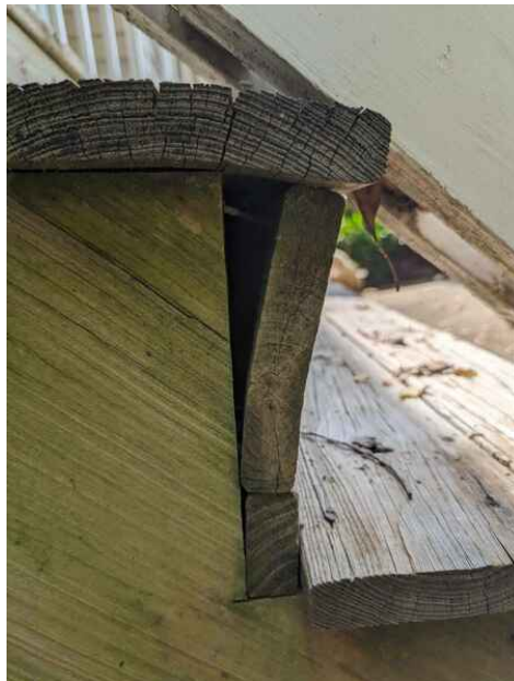
Step Pulling away from Stringer
