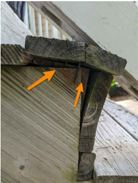
Corner of Stringer is broken loose and step is pulling away.
