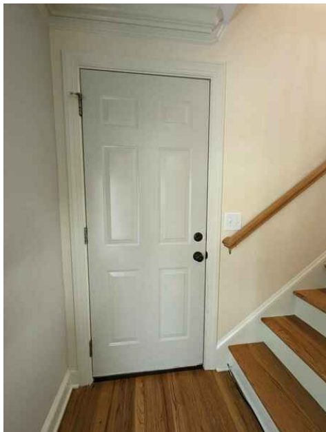
Door leading into garage does not have self closing hinges.
