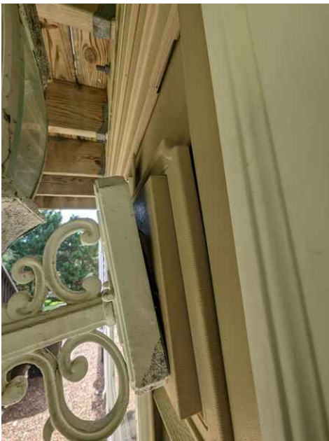
Light fixture on rear of house is pulling away from wall
