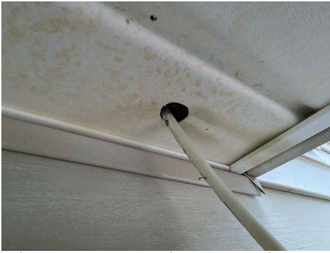
Where propane gas line enters the house should be caulked.
