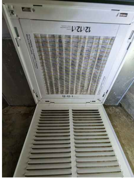
Filter at main air handler
